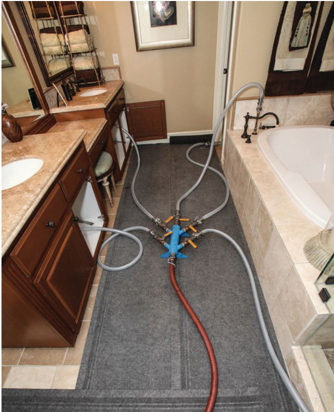
Most customers prefer pipe lining to traditional pipe repairs because pipe lining preserves their home or building, saving them money, time and hassle.
