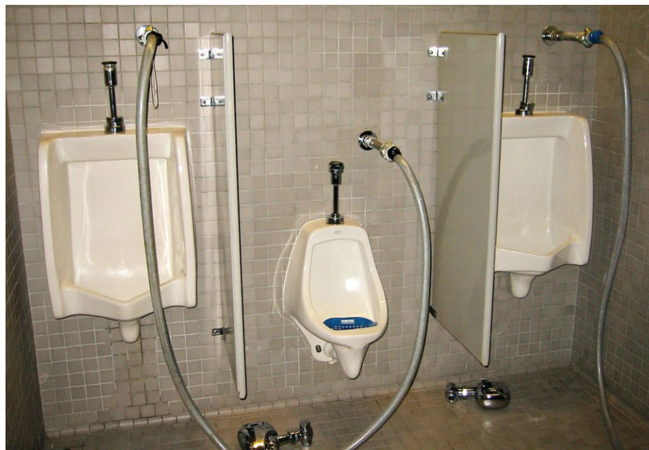
Pipe-lining technologies such as ePIPE, used in this picture, reduces disruptions to normal business activity in commercial properties.
